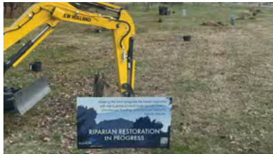
Over 800 trees and live stakes are planted to armor streambanks at this site in Springdale.
