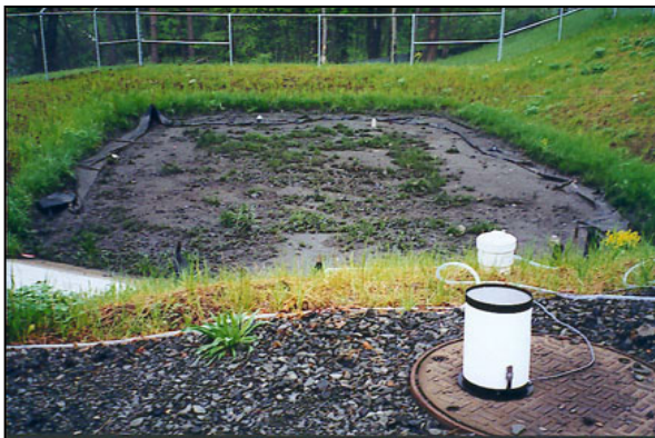
Surface Sand Filter
