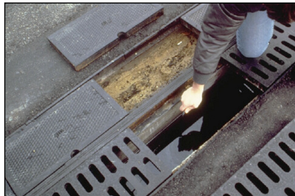
Perimeter Sand Filter
