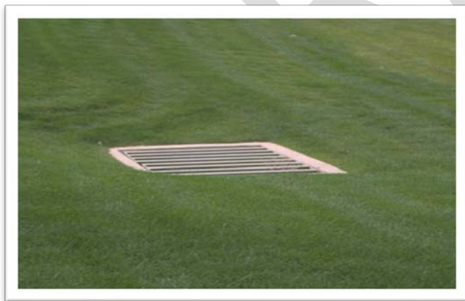
Photograph 3.6-2. Inlets frequently need maintenance.
