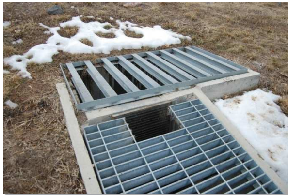
Photograph OS-4. Maintenance access to the water quality trash rack was compromised by the location of a secondary trash rack on this outlet. This may have been included as a safety rack or as additional protection from clogging. The owner modified the structure for better access. A safety rail would have been a better solution.
