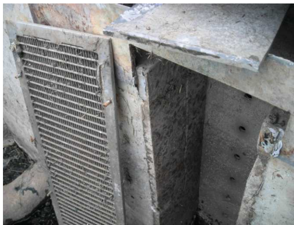
Photograph OS-2. This trash rack could not be properly
